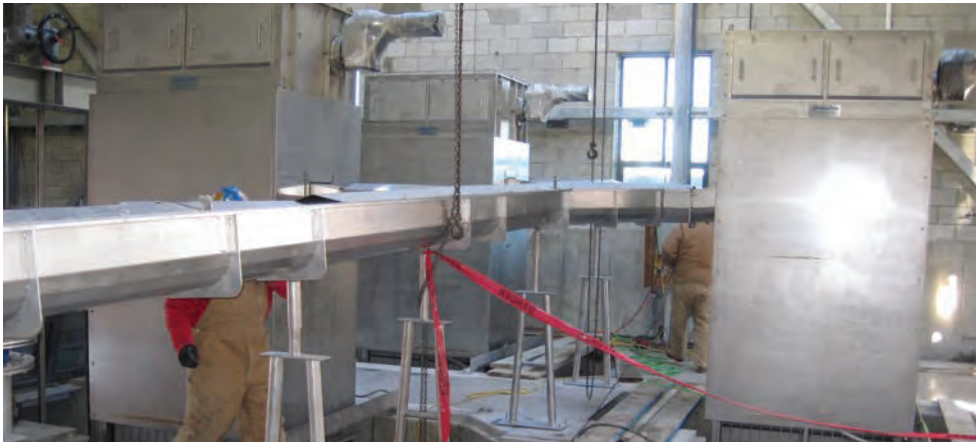
Three screens feeding into common sluice at plant during commissioning.
