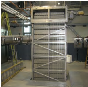
Screen shown at plant with covers removed.
